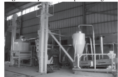
Fig. 13 Klapsho biofuel processing unit
