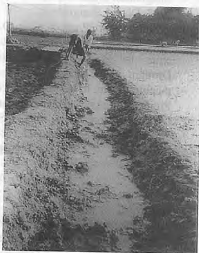
Fig.6(a) Unlined, uncompacted, irregular shaped canal.
