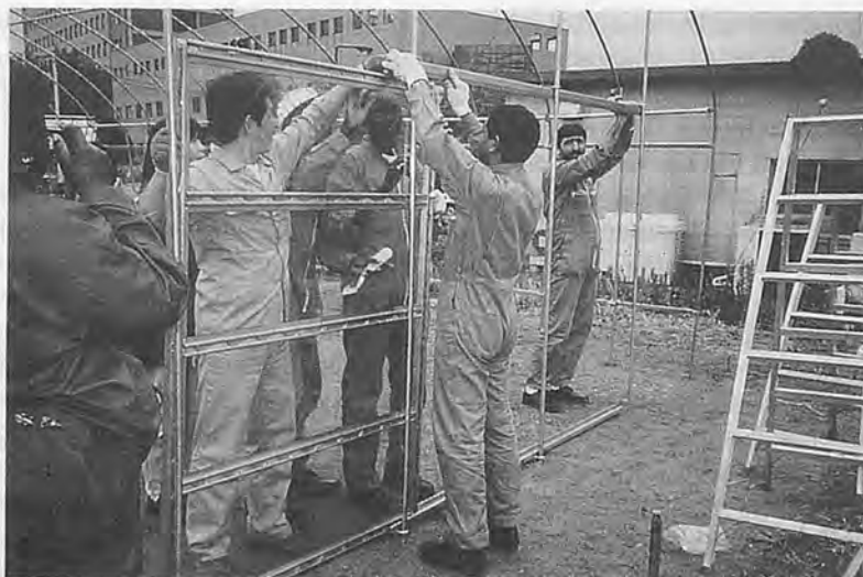
Fig. 1 Trainees are enjoying constructing a plastic house. It is one of important practice program in this training course conducted at Osaka Prefecture University.
