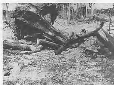
Fig. 2 A plot (BNW) bulldozed not windrowed. Knocked down trees cross-cut, packed and burnt.
