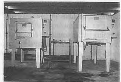
Fig. 10 View of heat treatment shop.
