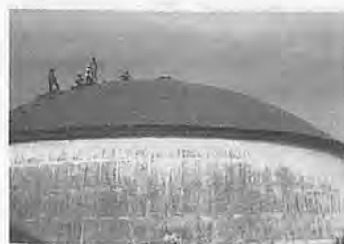
Fig. 10 Dome-shaped reinforced cement concrete silo in the Food Corporation of India, Borovli, India.
