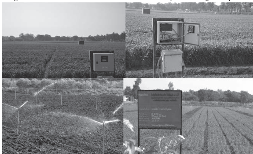
Fig. 3 Real time soil moisture sensor based automatic sprinkler irrigation system
