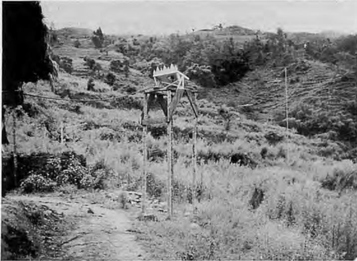
Fig. 1 Solar panel at Phikal Farm with broadband antenna in the background
