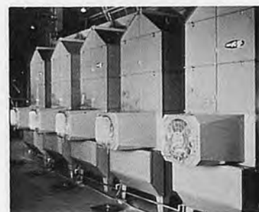
Isshingo "Rice-Con" Grain Drying Plant
