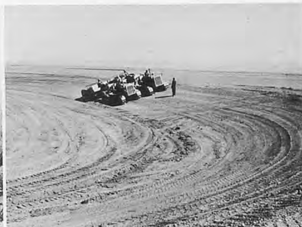
Photo.4. Iran. As Photo.3. The finishing stages of the construction of an irrigation water storage reservoir.
