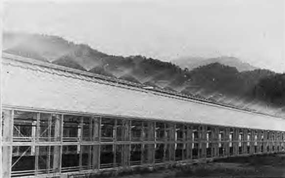
Photo 6. Rooftop water sprayers in operation
