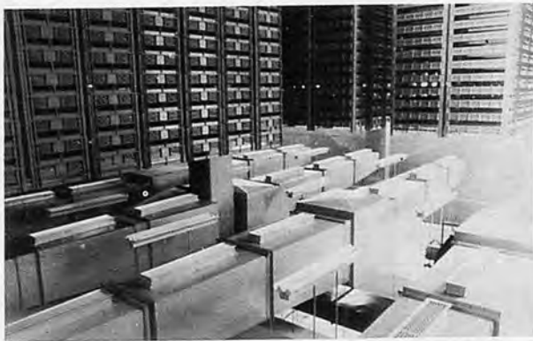
Photo 1. Bulb dry storage room with ducts and drying racks equipments are thus installed.
