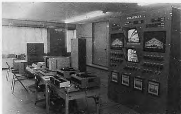
Photo 3. Central control panel (right)
