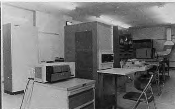
Photo 4. Central control room with appropriately laid-out equipments
