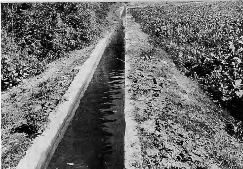
A field water course lined with brick masonry. Lining with suitable materials practically eliminates conveyance losses of irrigation water.
