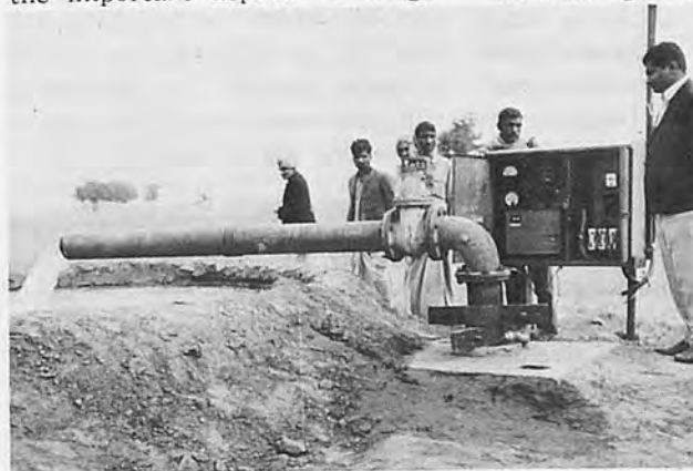
A submersible pump installed in a tube well drilled to over 300 metres depth in Hissar district of the State of Haryana. There has been a breakthrough in ground water exploration through open wells and tube wells since the advent of the green revolution.
