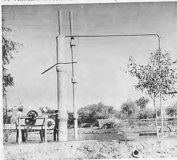
A high-head pump stand and vent pipe installed at the head end of an underground pipeline water distribution system in a hilly tract in the Rupar district of the State of Punjab. Note the pump delivery pipe feeding the line through the pump stand. Underground pipeline irrigation distribution systems are becoming increasingly popular in areas irrigated by wells.
