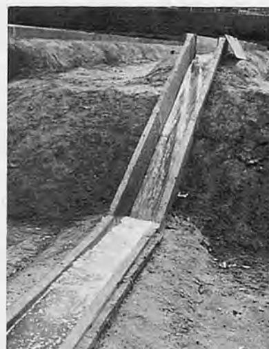
A chute spillway constructed with precast concrete channel sections is used to convey water down to a lower adjoining field at non-erosive velocity. Note the check gate installed at the inlet of the spillway.
