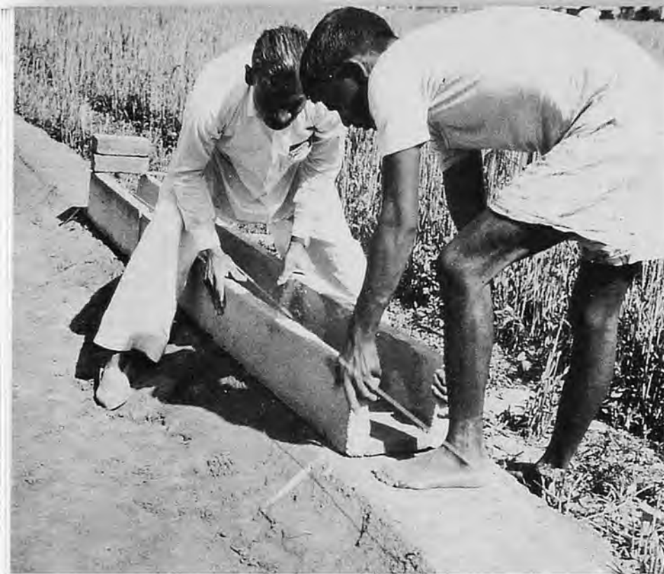
Laying precast concrete channel sections for the efficient distribution of irrigation water on the farm.
