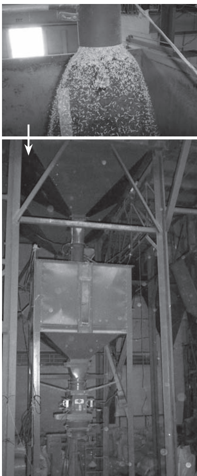
Fig. 4 The STM'S BWC attached to the hopper of seed processing plant
